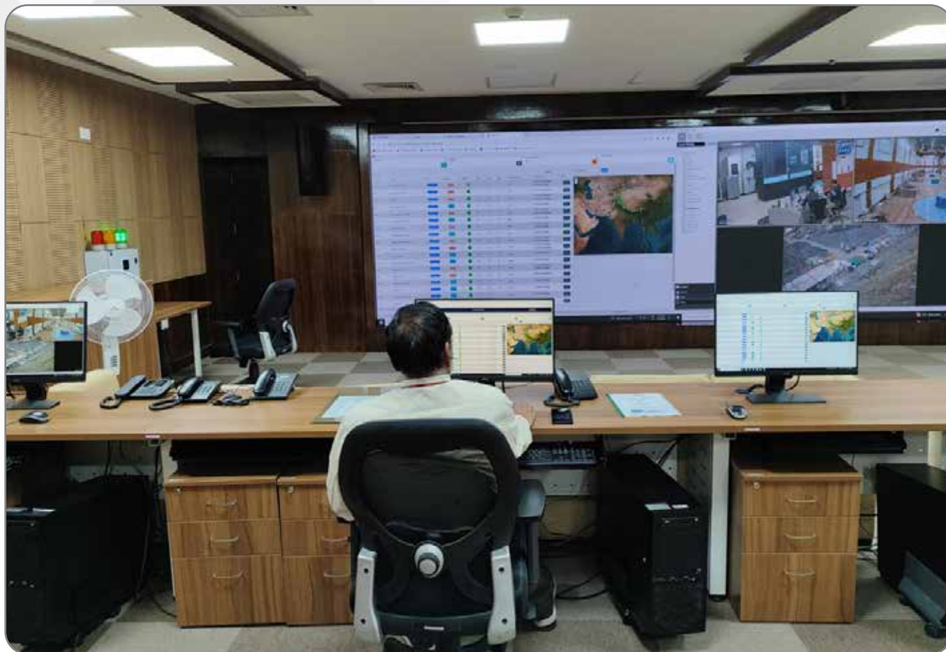
Master control room for EWS at NHPC, Faridabad
