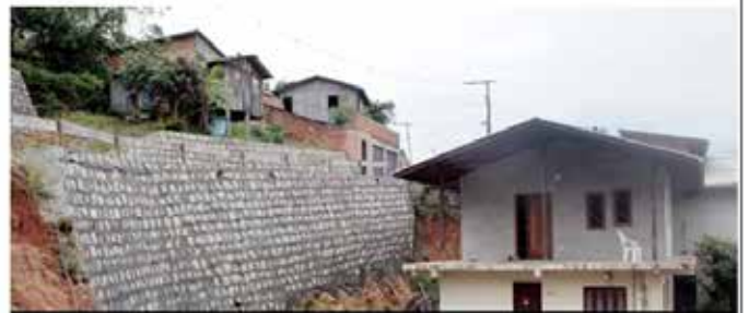
Slope Containment at Caiera Community
