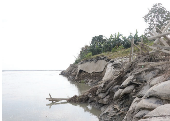
Figure 15.(a) Destroyed sandbags
